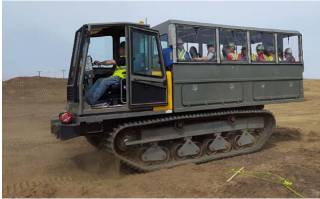
Figure 4. The Terramac RT9 crawler carrier hauls a crew, tools and the days supplies to a remote pipeline location.
