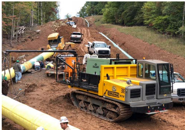
Figure 5. A compressor on tracks easily moves up and down the ROW as needed to provide services for multiple stages.
