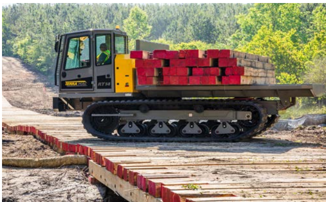
Figure 1. The Terramac RT14 crawler carrier with flatbed lays mats on a pipeline ROW.
