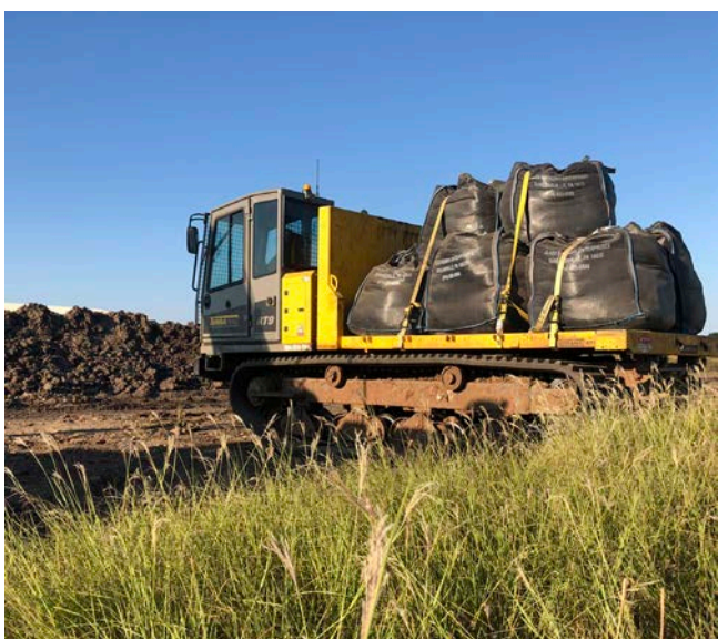
Figure 2. Hauling large sandbags up steep terrain requires a Terramac RT9 crawler carrier to get the job done.
